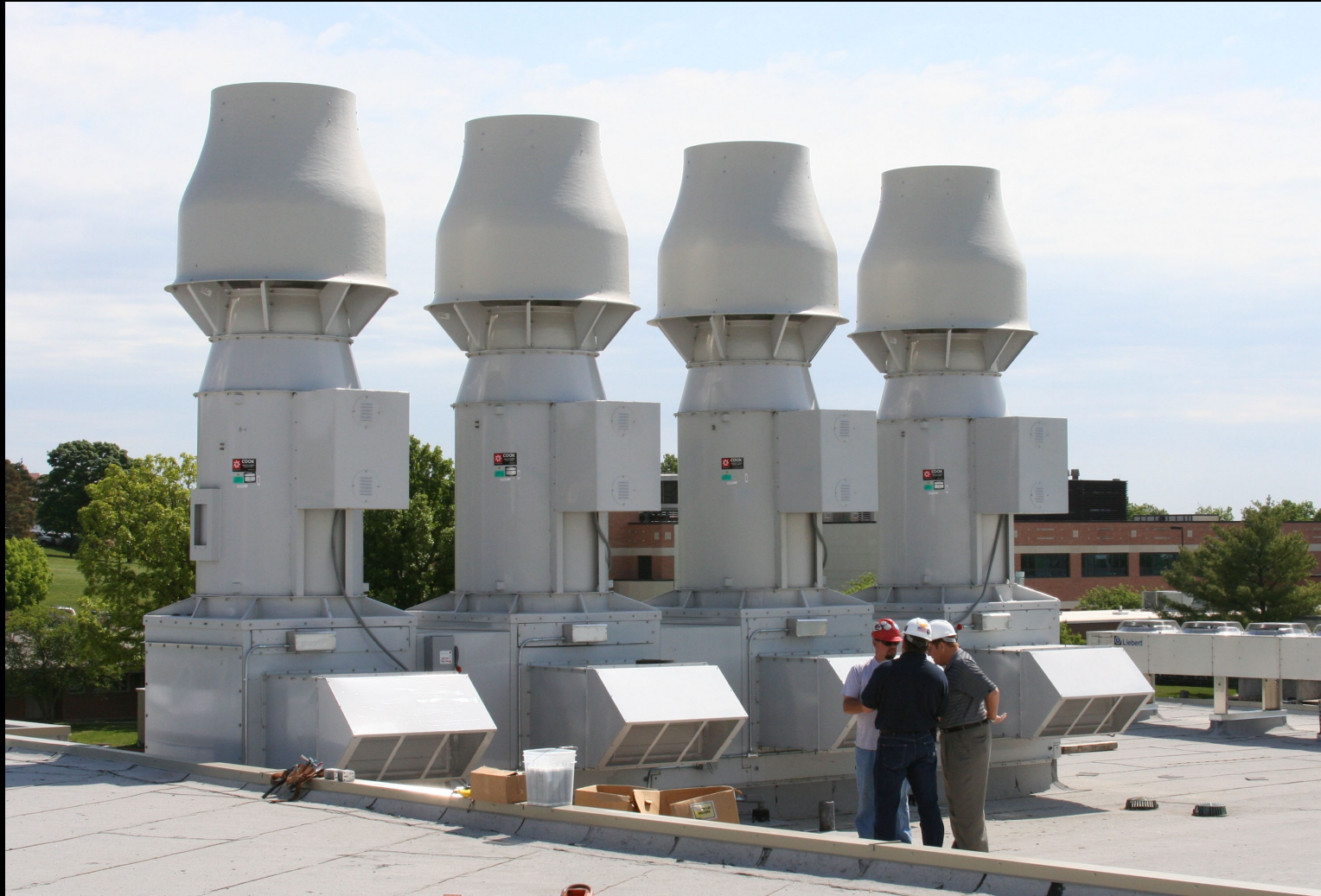
Multiple Lab Fans on common plenum
